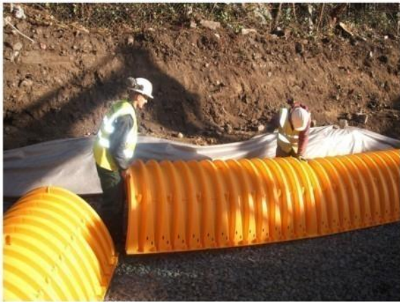
6. Lay Chambers as per drawing. 300mm clearance required from excavation edge. 150mm clearance required between chambers for stone. Spacers to be used.
