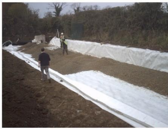
3. Lay pre-wrapped perforated pipe on Geotextile base. This pipe is to drain bottom layer of stone
